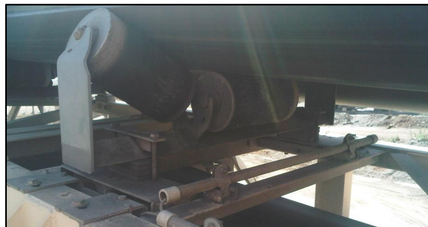
Previously installed weightometer frame
