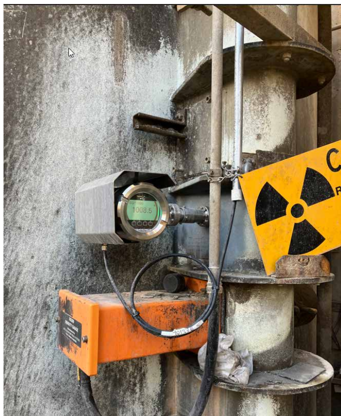
Fig. 1: The Rhosonics SDM installed alongside a radiation-based density meter
