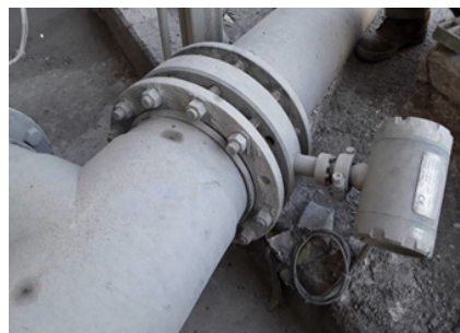
The SDM after four years of operating
